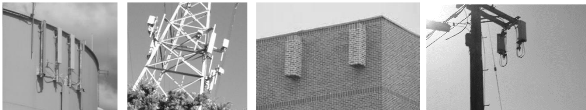
Examples of Flush Mounted Wireless Communication Facilities
